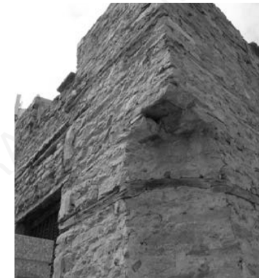
Undercut, chamfered corner
