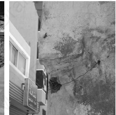
Undercut, chamfered corner
